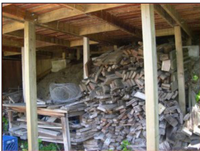
No deck, regardless of the material used to build it, would be safe if this amount of fuel beneath the deck caught fire. Even decks that may have a noncombustible surface, such as concrete, use lumber and timbers for structural support and those materials can catch fire.
